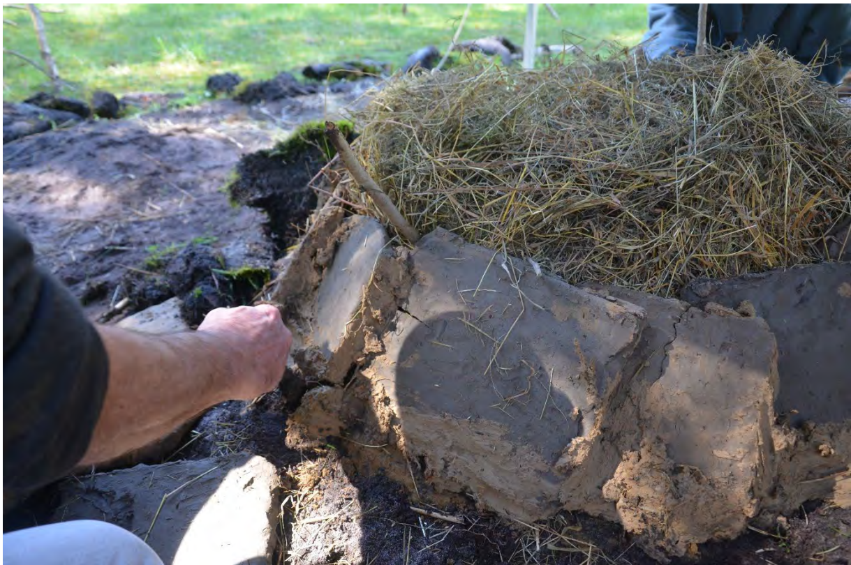
Fig18. Slabs for the dome being laid on the hay above the pots.
